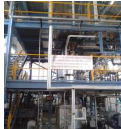
Multi feed/ multi chemical lignocellulosic ethanol pilot plant
