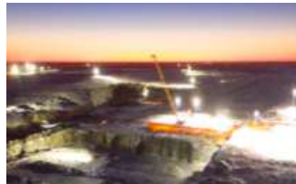
Keeyask Generating Station 695 MW
